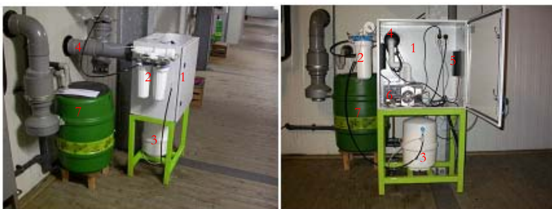
Illustration 1 Set up of Contronics humidification installation in this test. Left the closed module when in use, right a view of the opened module 1) gas-tight system cabinet 2) water filter unit 3) filtered water storage vat 4) combined supply room air / discharge humidified air 5) RH sensor/control DRZ-43 6) Ultrasonic humidifier HU-25 7) collection vat for measuring melt water from evaporator in the room (part of the regular room installation)
